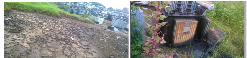
GOFA MAIN STORE SPILLED OIL AND CONTAMINATED SOIL
