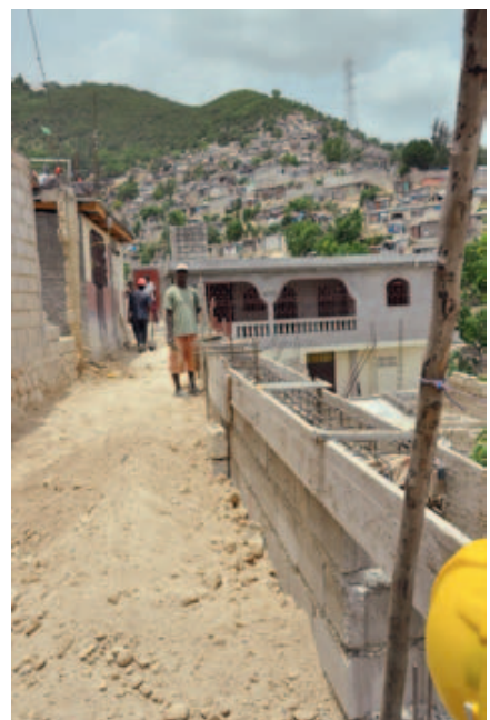
Paved Road as Part of Rehabilitation Project in Haiti (Photo by UNDP)
