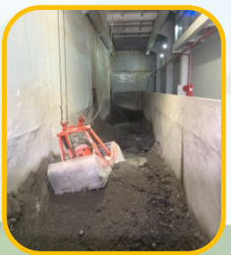
Ash collection and treatment system
