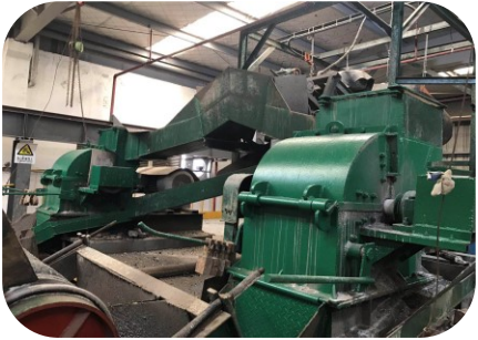
Bottom ash breaking equipment
