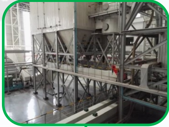
Flue gas treatment system
